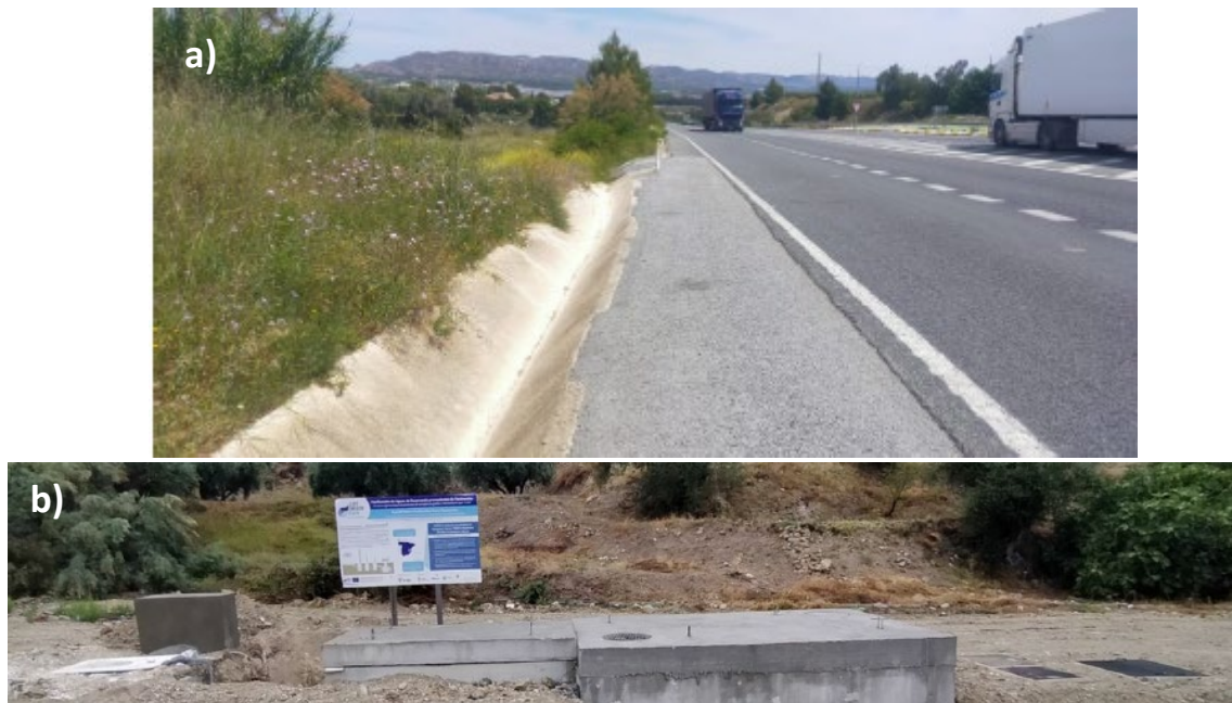
Figure 3. Porous photocatalytic pavement in Calasparra pilot (a) and treatment system (b) .
